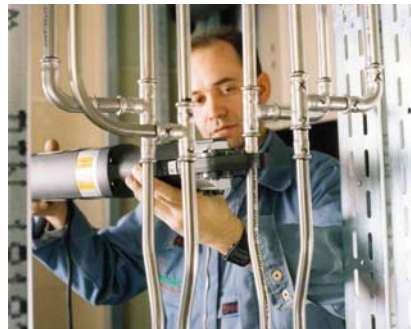
Stainless steel plumbing
