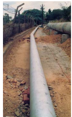
Raw water handling, India
